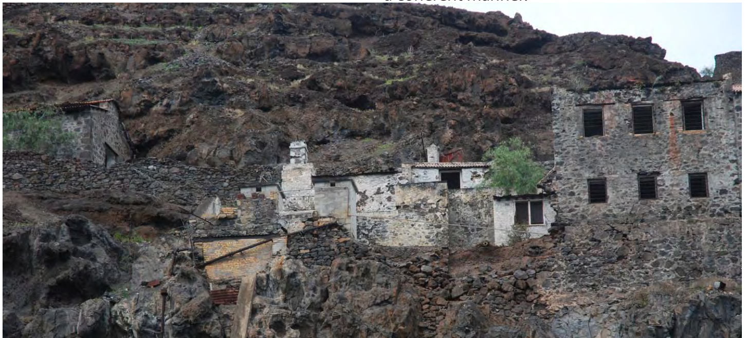
Some Sites Have Become Difficult To Access Due To Collapse, Urgent Works Are Needed
