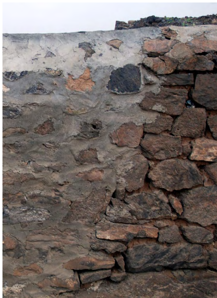
Before And After, Rather Unsympathetic Hard Cement Pointing, This Sort Of Repair Is All Too Common
