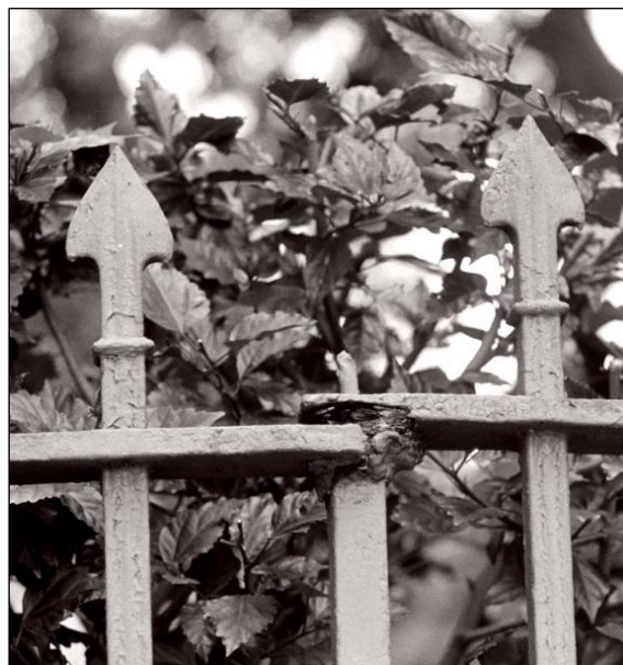
FIGURE 42: Public Gardens railings needing repair
