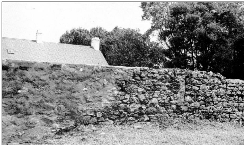
FIGURE 6: Walling – unsympathetic repairs – Bertrand's Cottage
