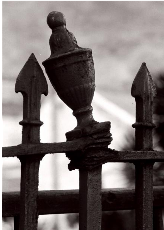
FIGURE 43: Public Gardens railings needing repair
