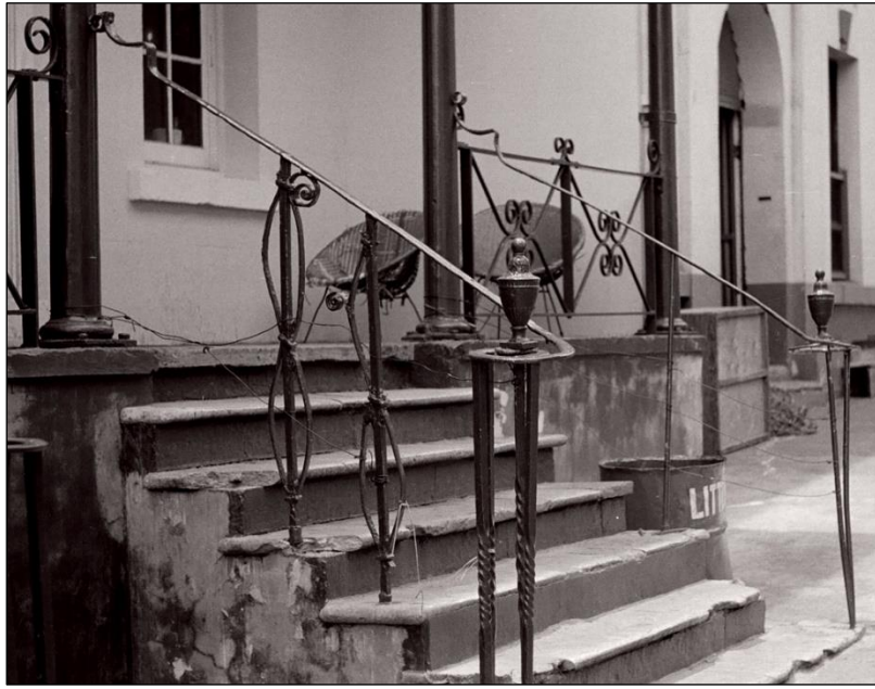
FIGURE 45: Dilapidated ironwork – Consulate Hotel
