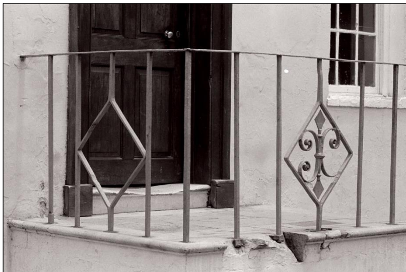
FIGURE 46: Dilapidated ironwork and stonework – W.M.C.A. Main St
